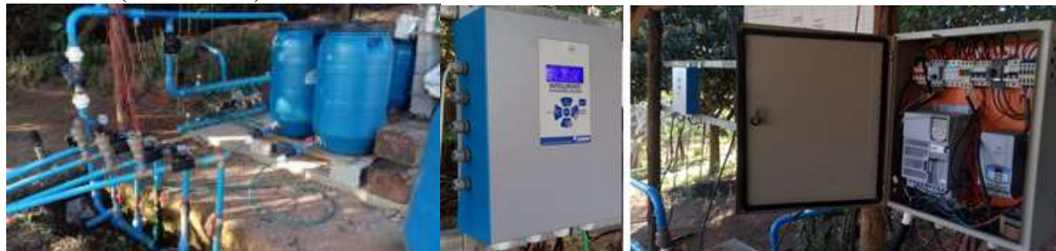
FIGURA 1. Equipamento instalado e em uso no campus experimental. Equipment installed and in use on the experimental campus.
